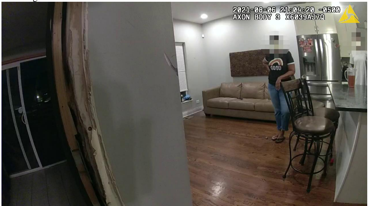
Figure 2. Close up of damaged door trim.
