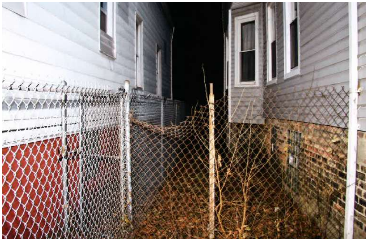
Figure 1. Photo showing the partially collapsed fence in the east gangway of [REDACTED] [REDACTED]
