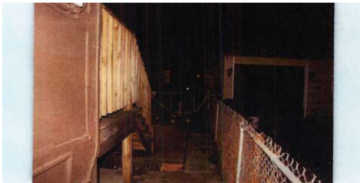
Figure 1: The view of the backyard from the south gangway of [REDACTED] Avenue. The wooden stairs and railing to the rear porch obstruct a complete view of the backyard from the gangway.
