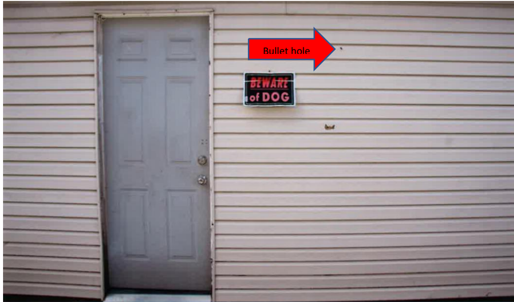
Figure 3: A suspected bullet hole on the exterior east wall of the garage at [REDACTED]
